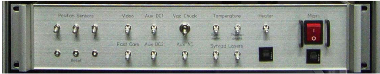
Figure 12 AAL power panel.
